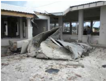
Samoa - Uplifted Slab-on-Grade
